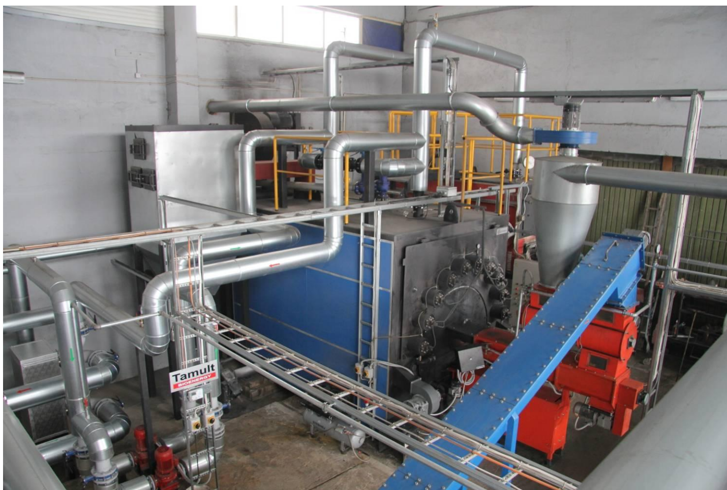
Figure 4.9 Danstoker biomass boiler at Lihula Boiler House (Photo: Ü. Kask)
