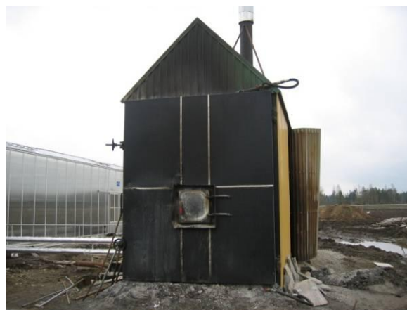
Figure 4.6 Boiler for burning round and square grass and straw bales (Photo: Ü. Kask)
